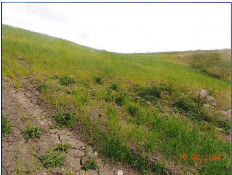
Photo 2 - Downstream embankment. The conduit is located below the boulders on the right side of the photograph.
