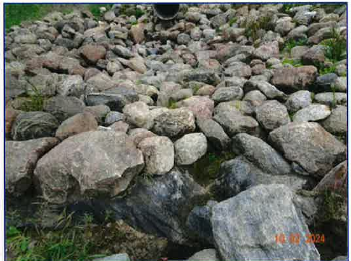
Photo 6 - Exposed geosynthetic in the riprap.
