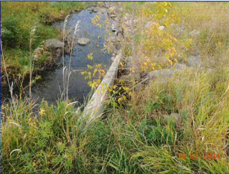
Photo 7 - Trees along the conduit outlet should be removed. There also appears to be a loss of soil along the culvert walls.
