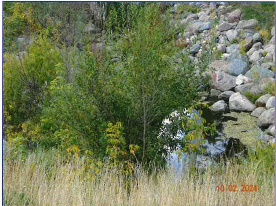
Photo 1 - Tree growth along the new conduit.
