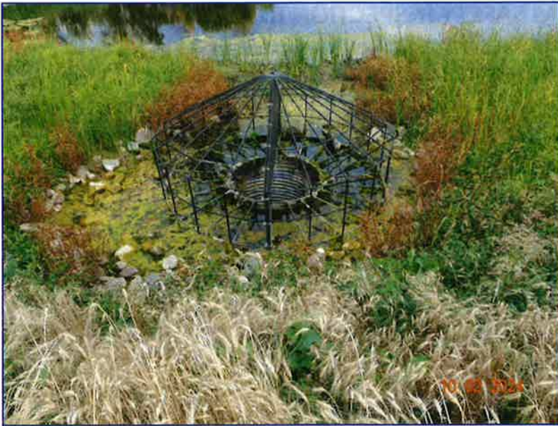
Photo 3 - Another view of the riser inlet.
