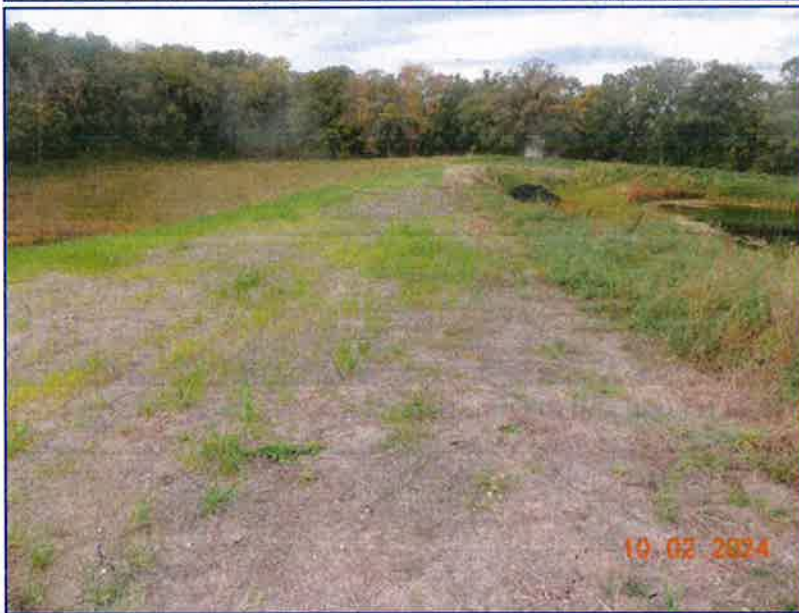
Photo 4 - Crest of the dam. A thin grass cover and minor soil desiccation was noted on the dam crest.
