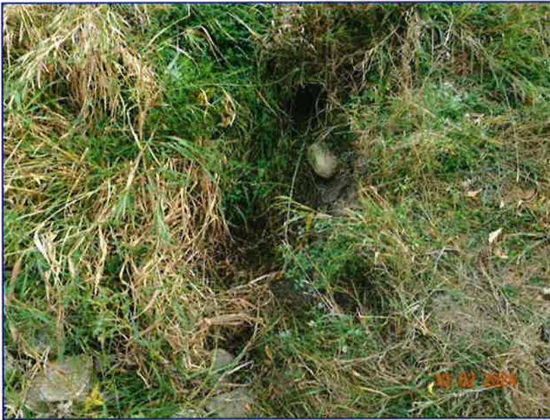
Photo 3 - Void in the embankment soil along the conduit. This is the same location as shown in Photo 2.
