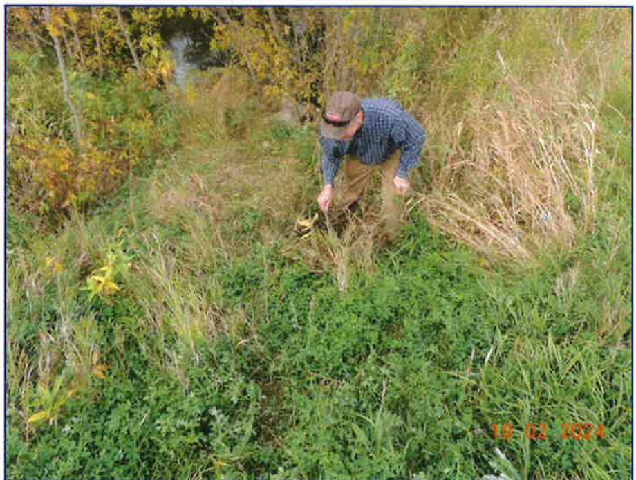
Photo 2 - Small embankment void near the conduit. Conduit outlet is at the waters edge near the top of the photograph.
