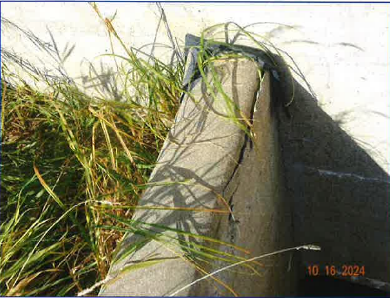
Photo 8 - Crack in the left concrete weir at the abutment wall.
