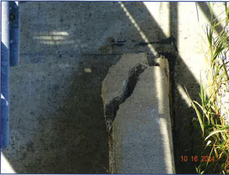
Photo 7 - Major crack with separation and displacement in the right concrete weir at the abutment wall.
