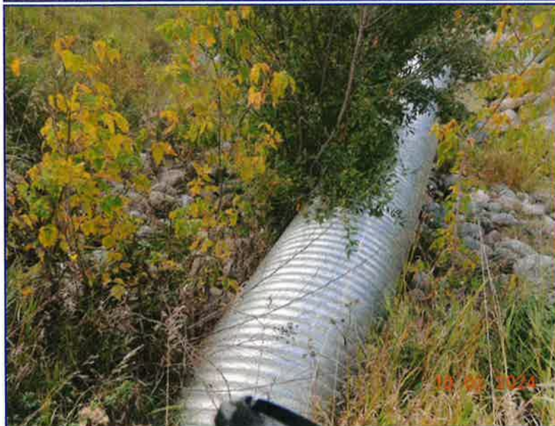
Photo 5 - Close-up view of the trees growing along the conduit.
