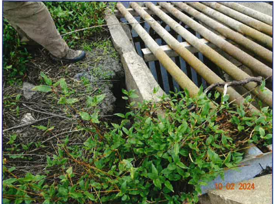
Photo 1 - Loss of soil along the right side of the low-level inlet.
