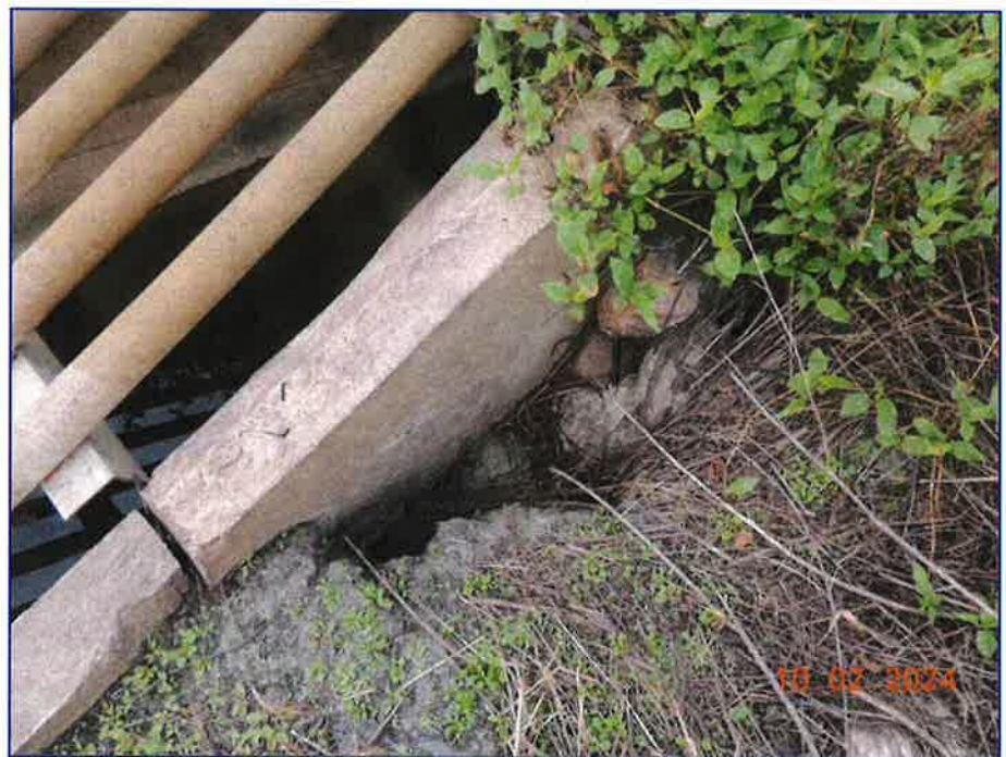
Photo 2 - Another view of the loss of soil on the right side of the low-level inlet. Note slight separation of the two sections of the box culverts.
